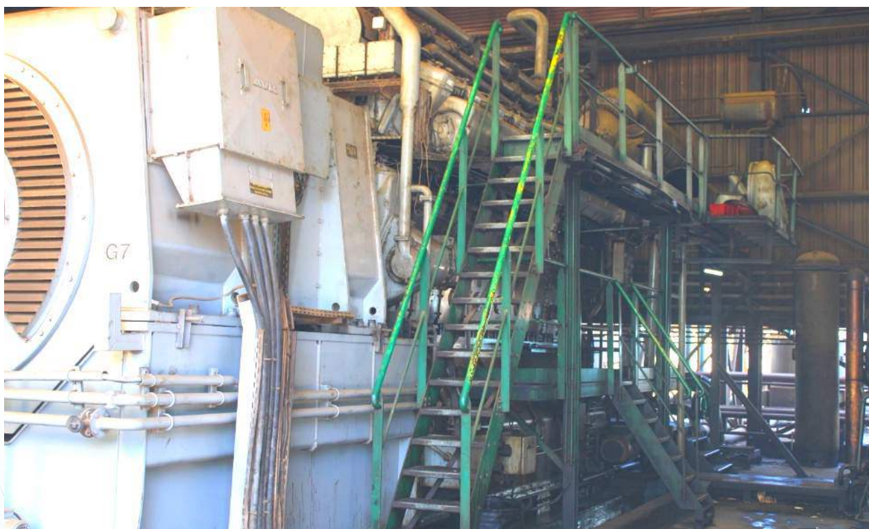
G7 at Kotu Power Station
