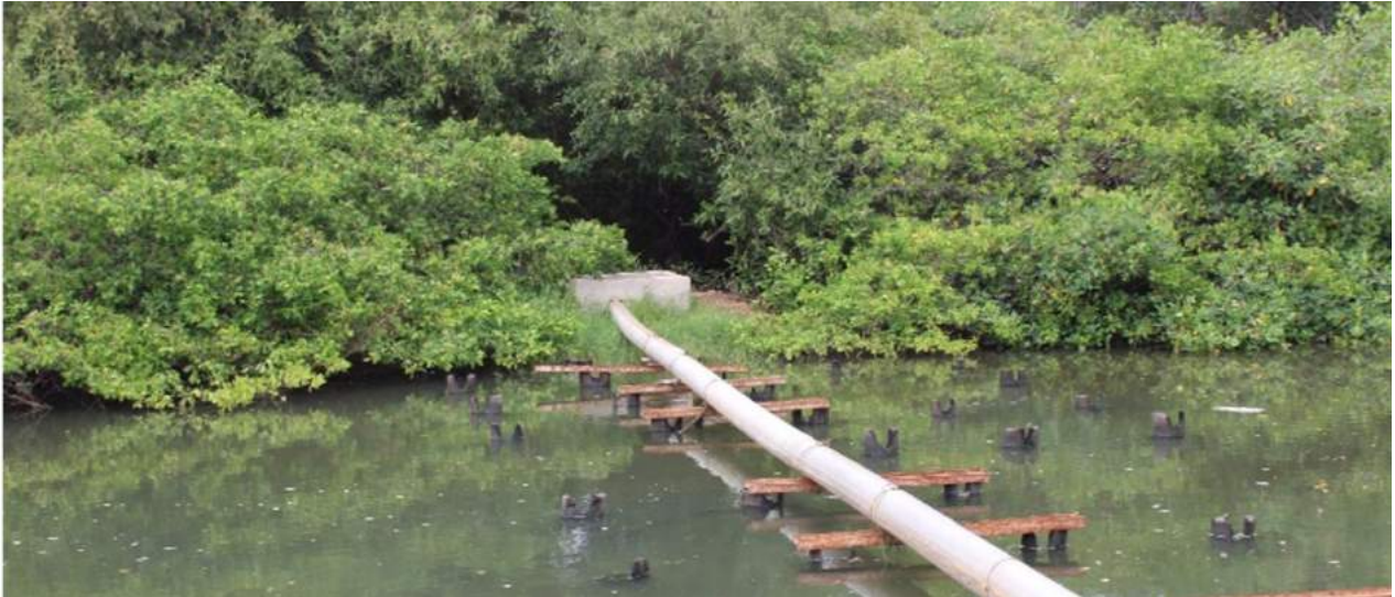
Sewage Pipe linking sewage pump #2 and the Lagoons in Kotu
