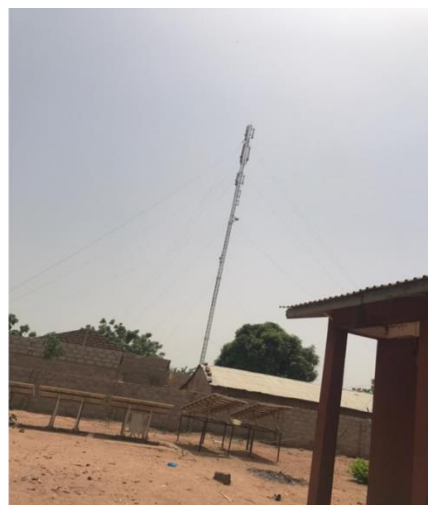
GAMTEL exchange station at Njaba Kunda, NBR
